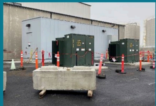
An additional electrical house was added to provide power to new facility infrastructure needed to support direct-feed low-activity waste operations.
