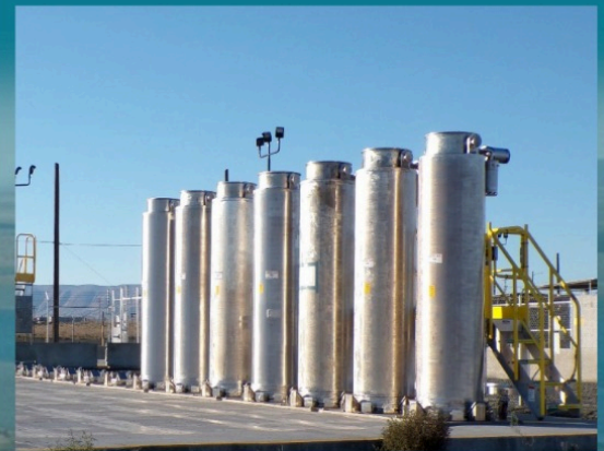
Spent ion exchange columns on the Tank-Side Cesium Removal System storage pad.
