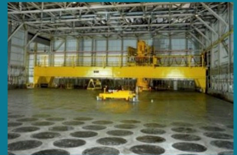
A crane inside the Canister Storage Building was used to place multicanister overpacks into belowgrade concrete vaults.
